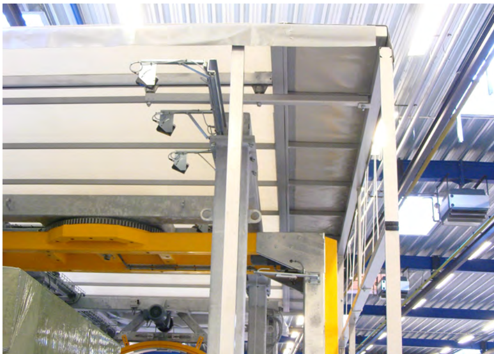
Trailer sides expanded to wrapping position. Note S3000 swingarm.
